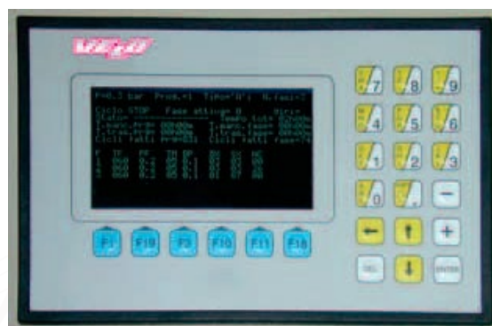
Quadro de controle – PLC
